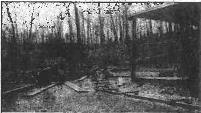
Johann, Harry & Robert constructing the wood lined water channel past the homestead.
