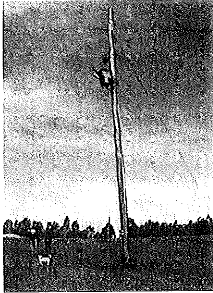
Plate 6: The 35kV transformer installed by the landowner located on the western boundary of the amendment site, approximately 315m from Brockman Highway.
